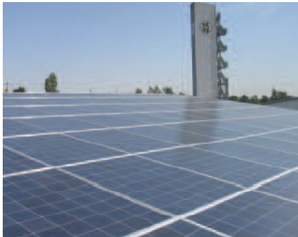
Large photovoltaic array Photo credit: Day4 Energy Ltd.
